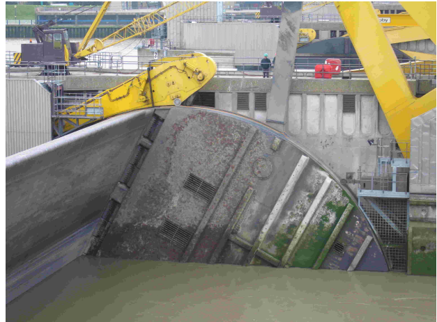
Figure 3 Z100 tracks on the Thames Barrier
